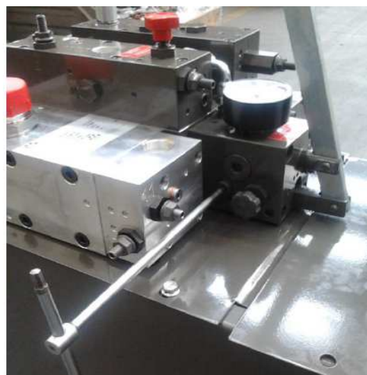
Pic. 17 – Installations with integrated HDU valve
